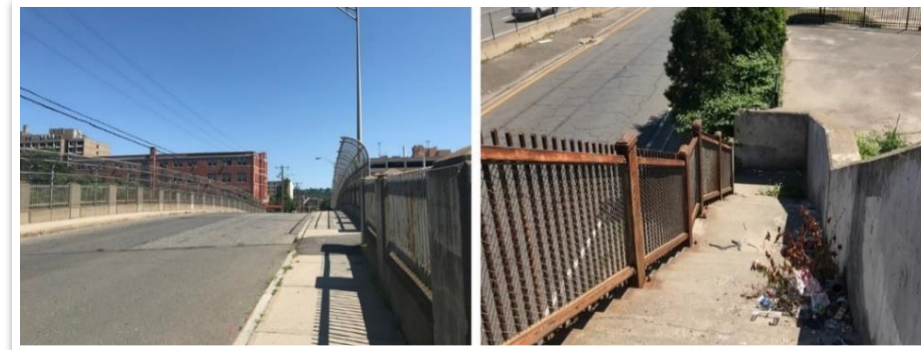
Figure 4-29 Photos of South Elm Street Overpass (Left) and McMahon Street Access (Right)
